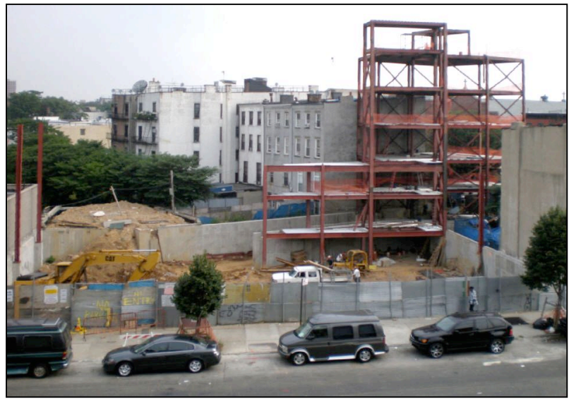
Foundation and steel construction were restricted to north portion of site for nearly five months, but project is now expected to finish on time and within budget.
